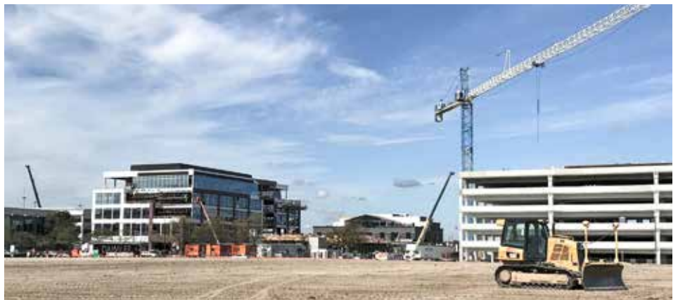
BUSY with Easton Towne Center's expansion project are George J. Igel & Company in the foreground and Wilhelm Construction and ALL Crane of Columbus in the background.
