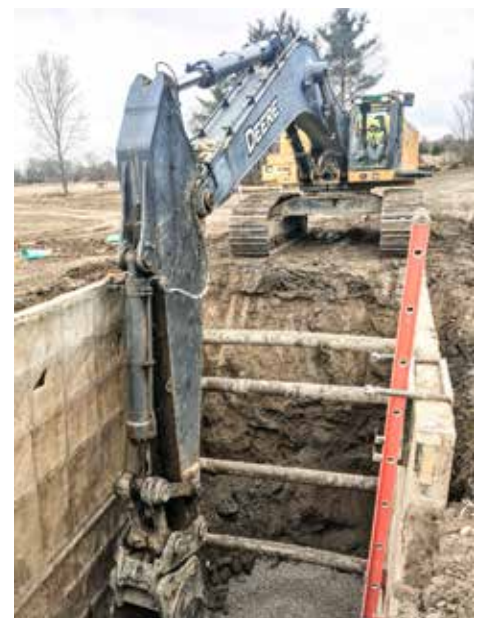
REPAIRING a broken water line on Wells Rd. in Delaware County for the George J. Igel & Company is Jerry Reeves.
