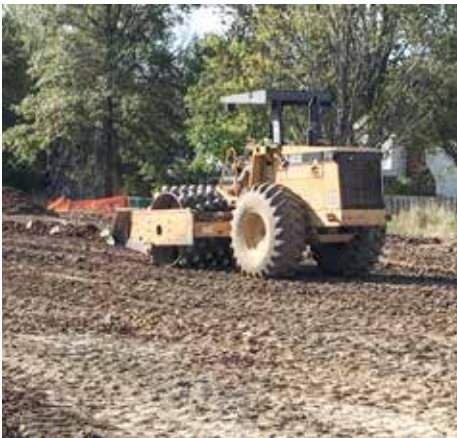
SITE work for a retirement home on Lorain Rd. in North Olmsted being done by Marous Brothers. Solomon Roscoe is operating the sheep's foot roller.
