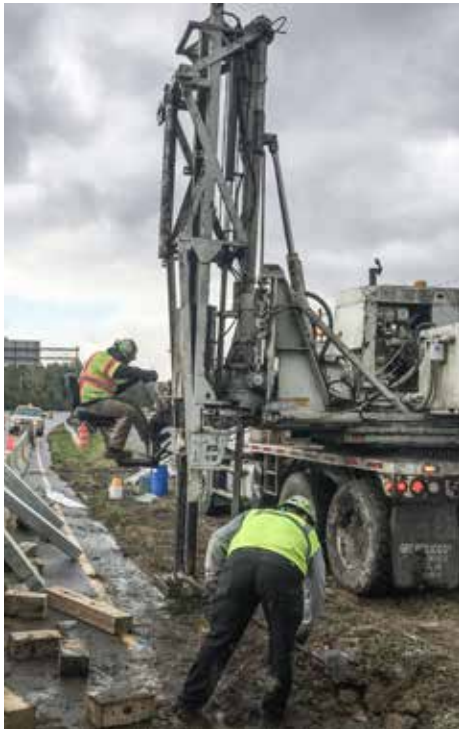
POUNDING guard rail posts on West Erie Ave. in Lorain is Lake Erie Construction, with Pilar Cabello operating the post pounder truck.
