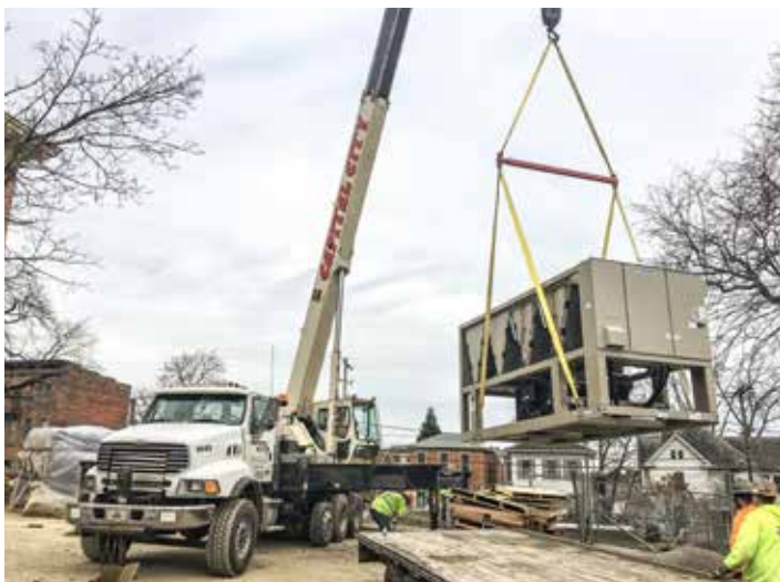
WORKING at the Delaware County Courthouse for Capital City Crane is Rick Roshon.
