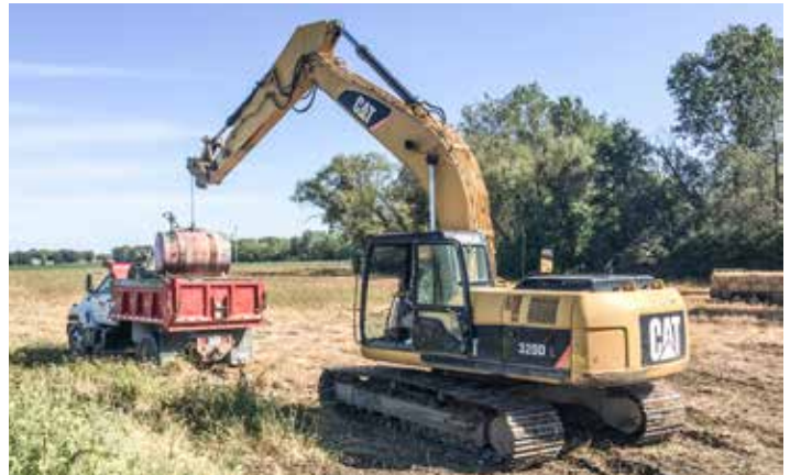
LOADING out after finishing up a bridge job on Billings Rd. in Castalia is Schalk Brothers. Donnie Saalman is operating the hoe.
