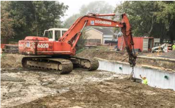
REPLACING a culvert on Adele Lane in Olmsted Falls is Schirmer. George Janosik is operating the hoe.
