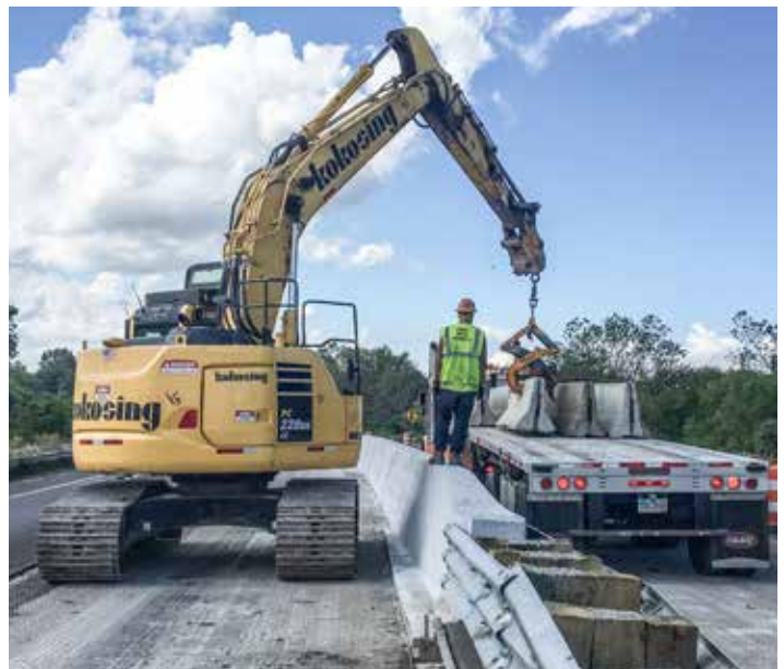
LOADING out barrier wall on S.R. 113 in Elyria is Kokosing. Steve Seidel is operating the hoe.
