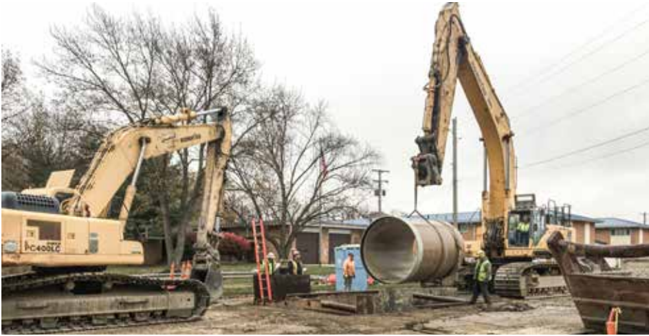
SETTING 78-inch sewer line on Abbe Rd. in Elyria for the 3rd phase of the east side relief project is Fabrizi. Billy Dezarn is operating the PC800 hoe and Brook Murray is the oiler.
