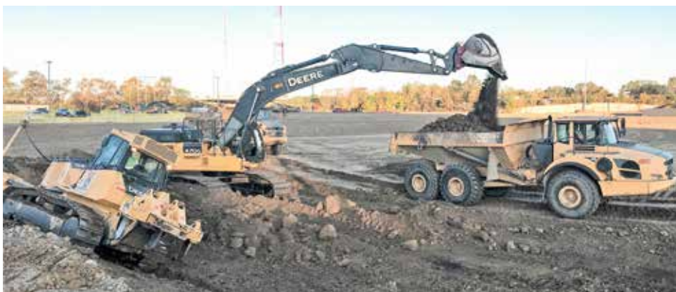
PERFORMING the mass excavation at the Columbus Crew stadium is George J. Igel & Company.
