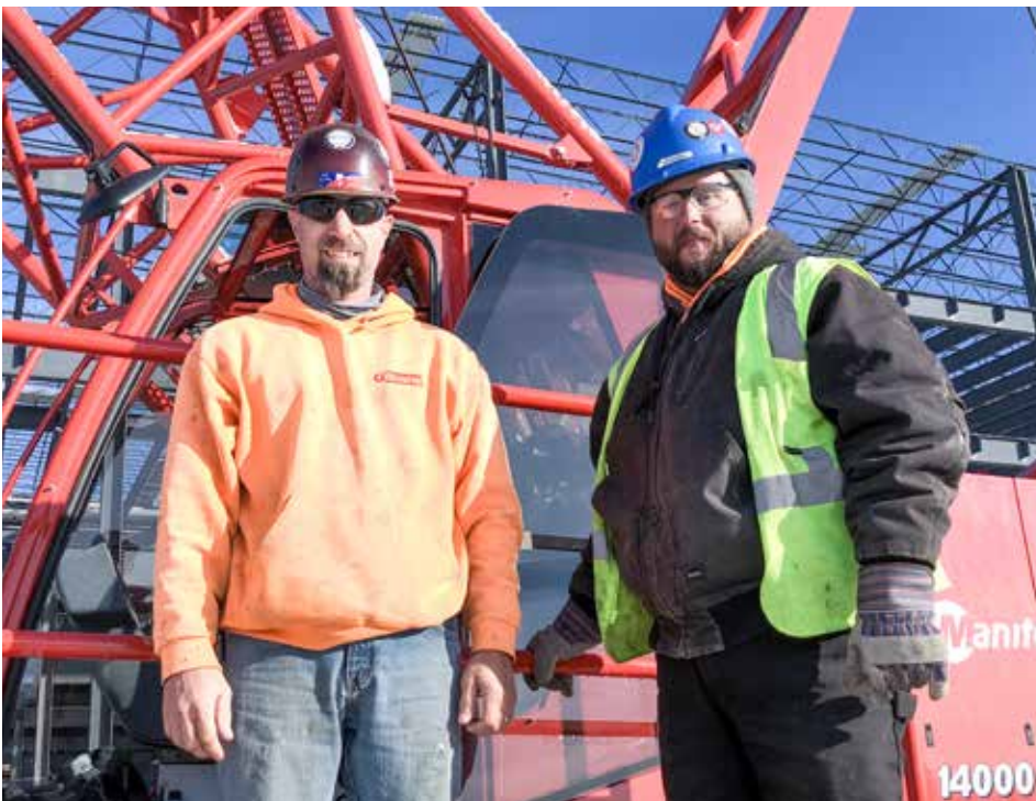
WORKING for Kelly Steel at the Amazon project in Summit County are (l-r) Matt Krause and apprentice Steve Vasko.
